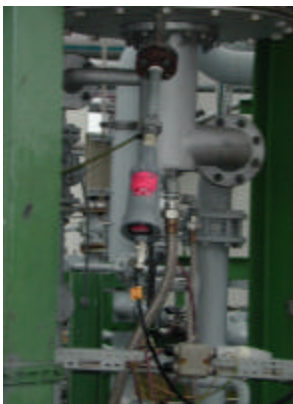
(Lower Flame Scanner)
