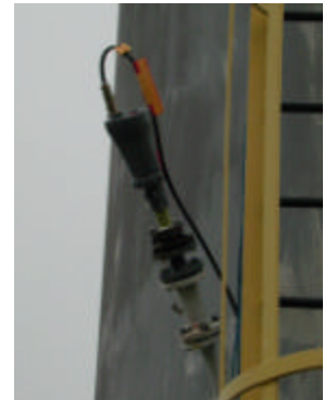
(Upper Flame Scanner)
